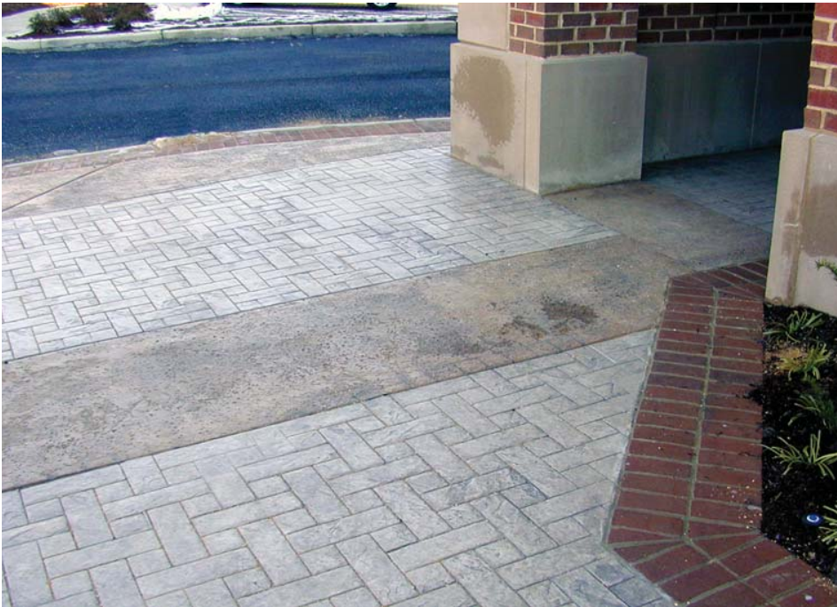
Clubhouse Plaza Paving utilizes cost-effective application of patterned concrete in coordination w/ Arlington Co
